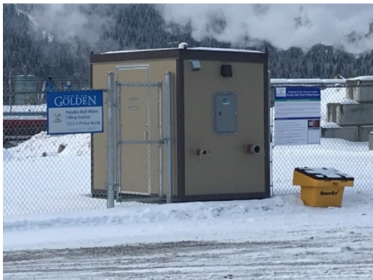
Potable Bulk Water Filling Station
